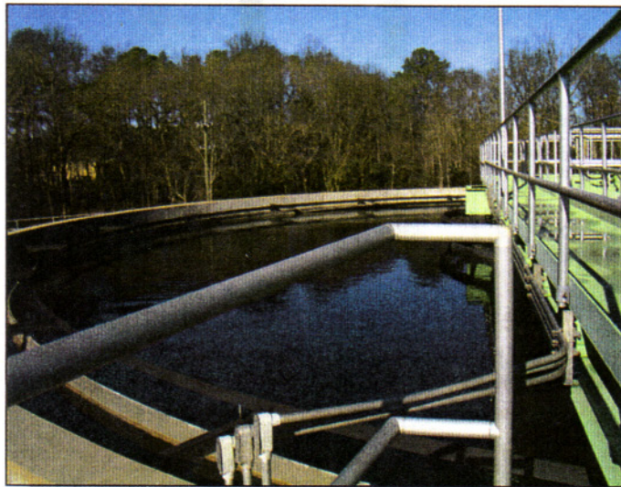
A view of the clarifier at the Alabaster, Alabama wastewater treatment plant, located in one of the fastest-growing counties in the country. Revere Control Systems photo
