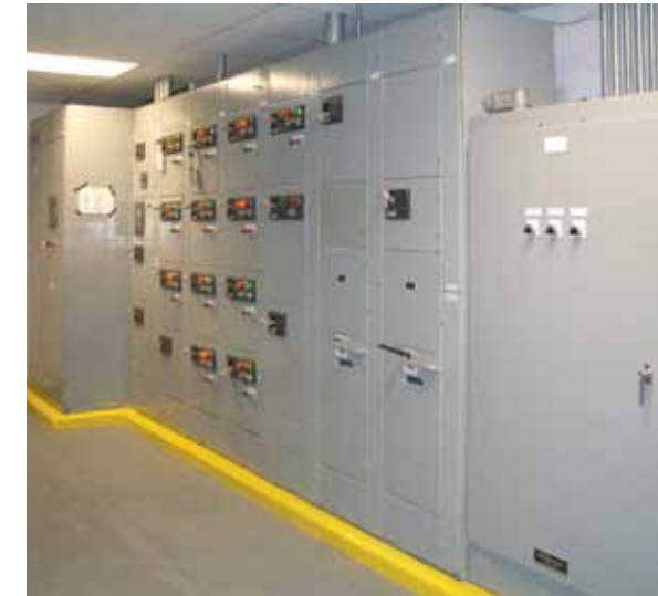
PLC panel (at right) automates the new treatment train, including pump station #1, oxidation ditch surface aerators, and submersible mixers. The panel is wired directly to the motor control center (remaining panels) which contains the motor starters for this equipment).
