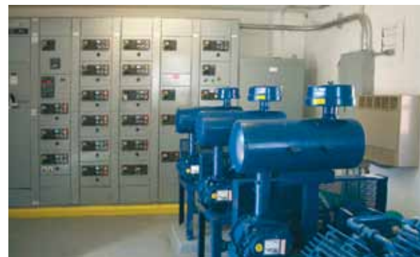
Pneumatic valve compressors (foreground) with Revere panels in the background.
