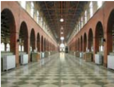
The main entrance to the filter building. Filters and their controls are lined up on both the left and right.
