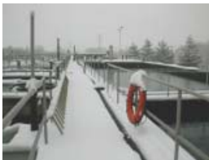
A rare Tennessee snowstorm highlights grit tanks (on the left) and flocculators.
