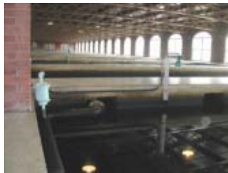
One of the filters showing the ultrasonic level transmitter that signals high and low levels to the filter controls.
