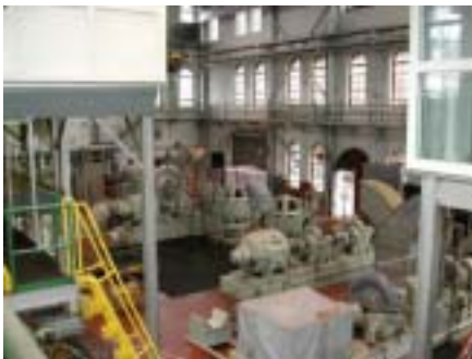
The main floor of the pump station building.
