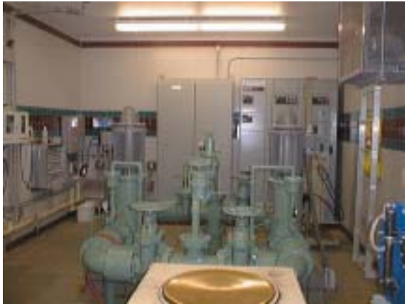
Inside permanganate building
