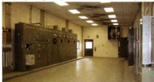
North and South control bay lineups.
