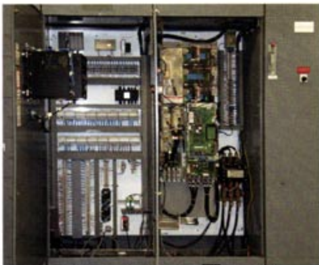
A PLC cabinet (left) and a drive cabinet for the North lineup.
