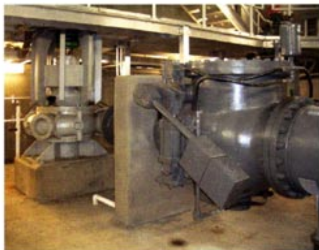
A pump and valve combination leading into the 42-in header pipe.
