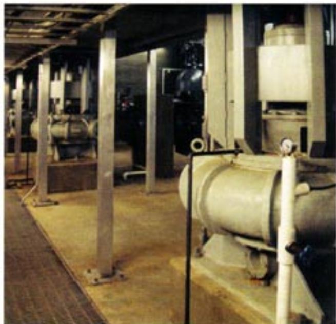
One of two dry wells showing the three Patterson pumps.
